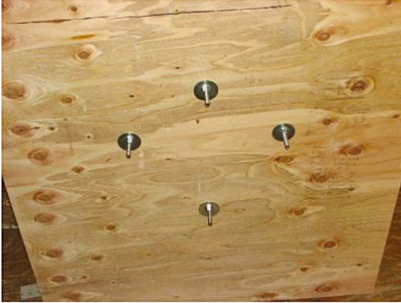
These are the carriage bolts poking thru the plywood and being held tightly in place by fender washers, regular washers and nuts.
