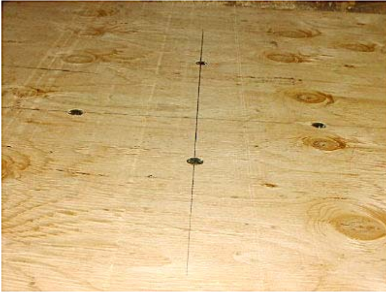
These are the carriage bolts that have been sucked into the plywood so that they are flush with the surface of the plywood.
